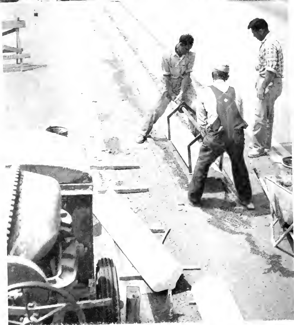
UPPER LEFT Unloading curb sections. UPPER RIGHT—Driving anchor steel for center divider. LOWER Setting section of center divider.
